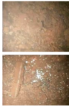
Status inside the pedestal (A2' investigation results)
