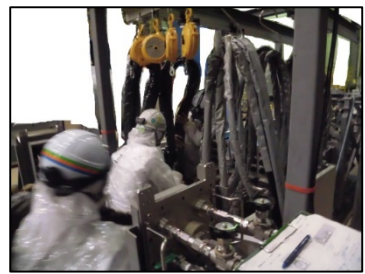
Status of wiring of the equipment
