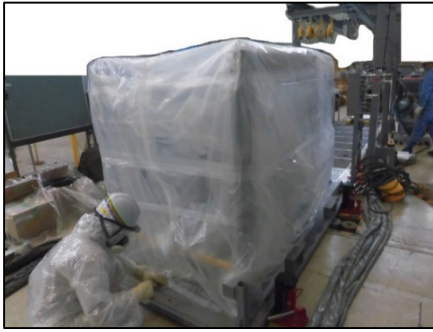
Status of the lid for preventing spread of contamination
