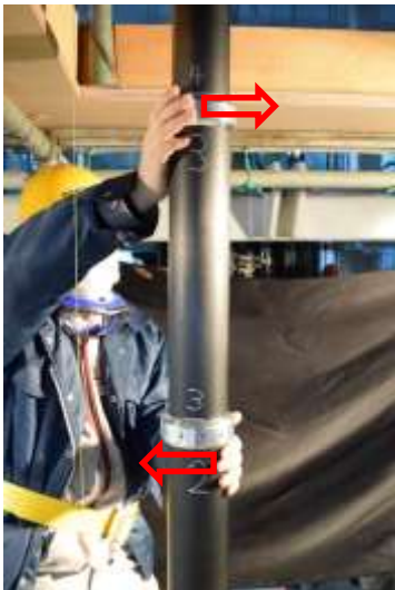
The bending direction force is being applied to the pipe so that the third stage pipe is inclined
