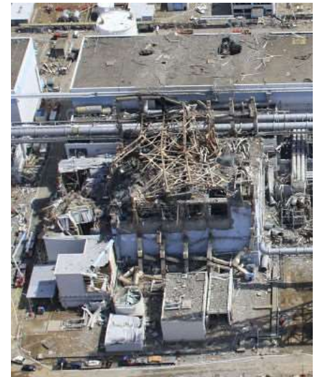
Just after Hydrogen explosion on 1F1&1F3
