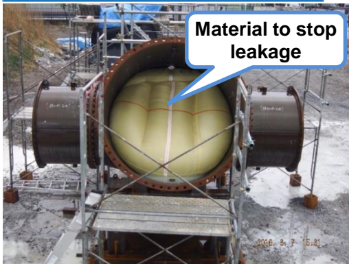
Water stop performance of the material was verified by using the full-scale test facility (outdoor).
