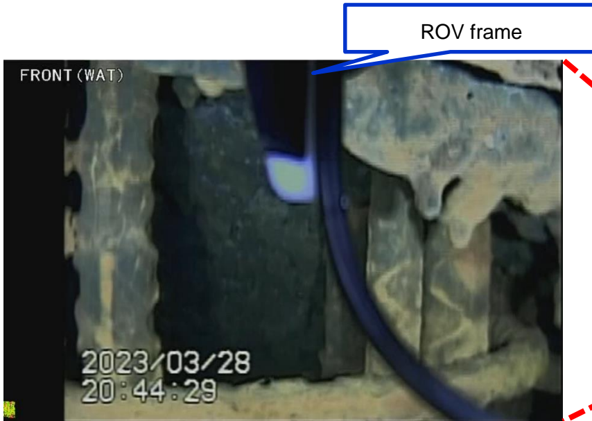
Photo 1: Concrete remains can be seen from the pedestal opening
